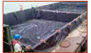
ACEContainer™ Geotextile Containers Fitting in Split Barge for Marine Structure Construction, Land Reclamation, and Dredging
